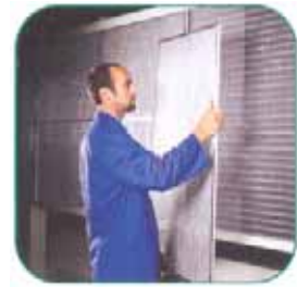
Filtermatten am Kondensator Condenser air filters
